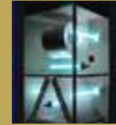
Internal UV lights, sanitizing drain pan, cooling coils, and internal components of the dedicated outside air units.
